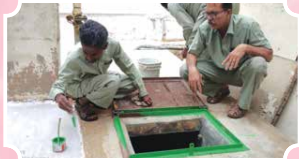
Water tank has been cleaned, painting of cover lid has been done at Head Office
